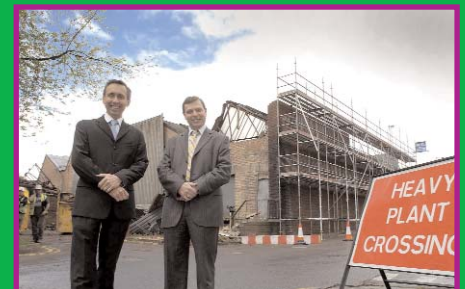
Tim Hurdiss (left) and Mike Jones in front of Coronet House before it was demolished.
